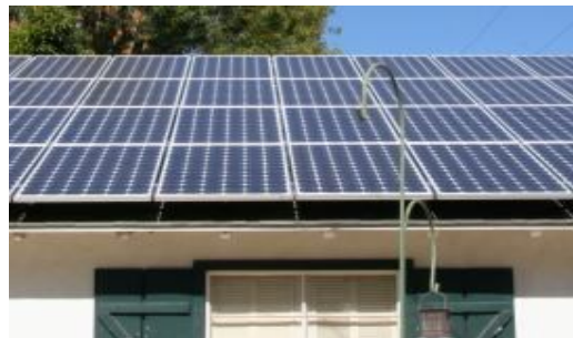
Fig 2. a roof mounted PV array.
